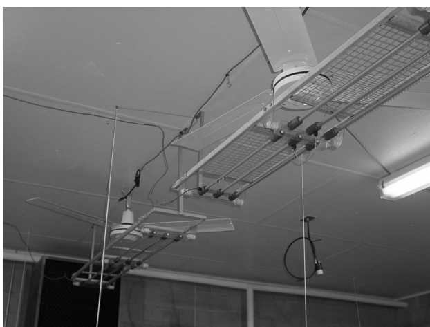
Figure 2. ESCS units suspended below the ceiling fans in the treatment room.
